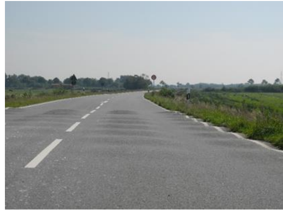
Figure 3 : Example of punching failure of low height embankment over rigid inclusions
